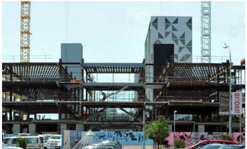
Cellular beams fabricated by HERA member Grayson Engineering in use at the Britomart Transport Centre's East extension
