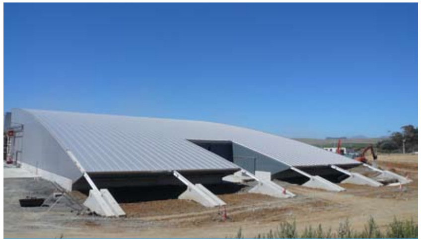
Yealands Estate Winery in Seddon, Marlborough nears completion in 2008. Designed by HERA member Structex, it is the first winery in NZ to comply with the GreenStar NZ Industrial rating requirements.
