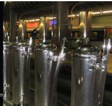
Stainless Steel air filters in the Britomart Transport Centre, Auckland
