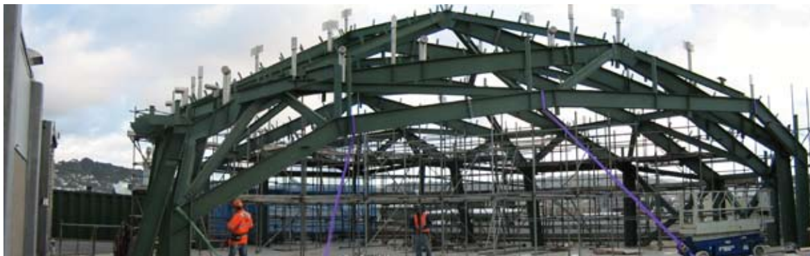
Wellington Airport International Terminal - 'The Rock', fabricated by HERA member Stevensons Structural Engineers
