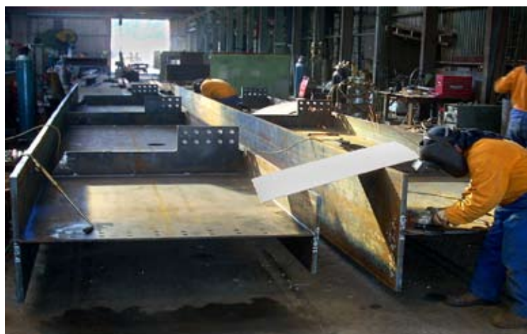
Fabrication of the main girder for the Contact Energy bridge by HERA member Eastbridge
