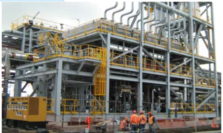
Staff from HERA member Fitzroy Engineering finalising installation of the 240 tonne MEG Regeneration Skid at the Kupe site in South Taranaki.
