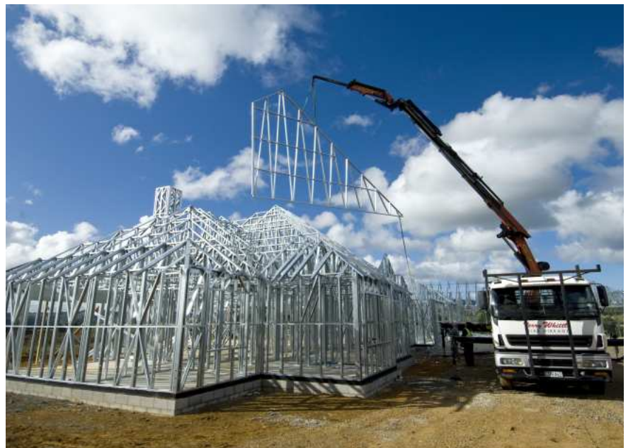
Efficiently erected light steel-framed house made from AXXIS Steel of HERA member NZ Steel
