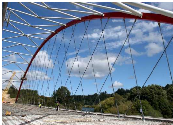
Fantastic view of the Waikato river bridge, designed by HERA members Holmes Consulting Group and fabricated by Tenix Group
