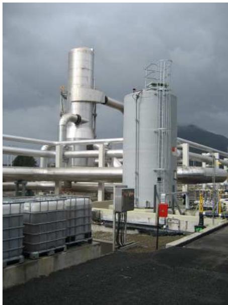
Pipes, vessels and cooling towers were fabricated locally by various HERA members for Mighty River Power's geothermal plant in Kawerau
