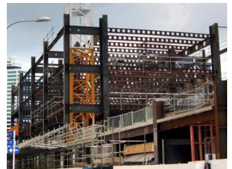
Steel work (featuring HERA member Grayson Engineering's Cellbeams) at the Britomart East one and two project, Auckland. The $11m project used approximately 3,000 tonnes of steel.
