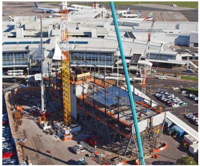
The Novotel at Auckland International Airport under construction by HERA members Hawkins Construction and George Grant Engineering (GGE), contains close to 600 tonnes of structural steel. The 40-tonne front entry canopy was assembled in their workshop in sections, broken down and re-assembled on-site. To lift this canopy into position, two 80-tonne cranes and a 150-tonne crane were used.
