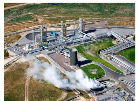
HERA member SKM was engaged as engineering designers for the steam separation system at Nga Awa Purua—a new 140MW, $430 million geothermal power station in Taupo. Nga Awa Purua houses the largest single shaft geothermal turbine in the world and provides enough electricity to power 140,000 homes (equivalent to Taupo, Rotorua, Hamilton and Tauranga combined).
