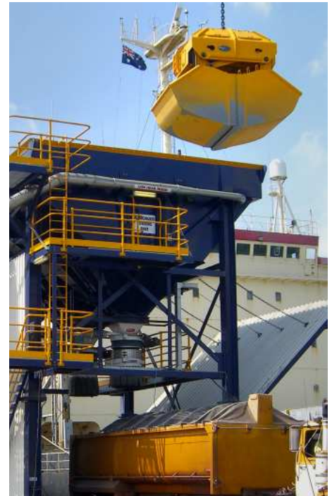
Page Macrae Engineering continues its export drive of bulk handling solutions which includes its Australian Bulk Handling Awards winning hopper-grab combinations. The photo shows the 10cum diesel-hydraulic grab and hopper in operation at Bunbury in Western Australia.
