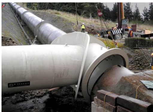
A 25-tonne section of a hydro power station penstock used to divert water to an irrigation scheme fabricated by HERA member Fitzroy Engineering for Trustpower's Highbank power station at the Rakaia River in mid-Canterbury
