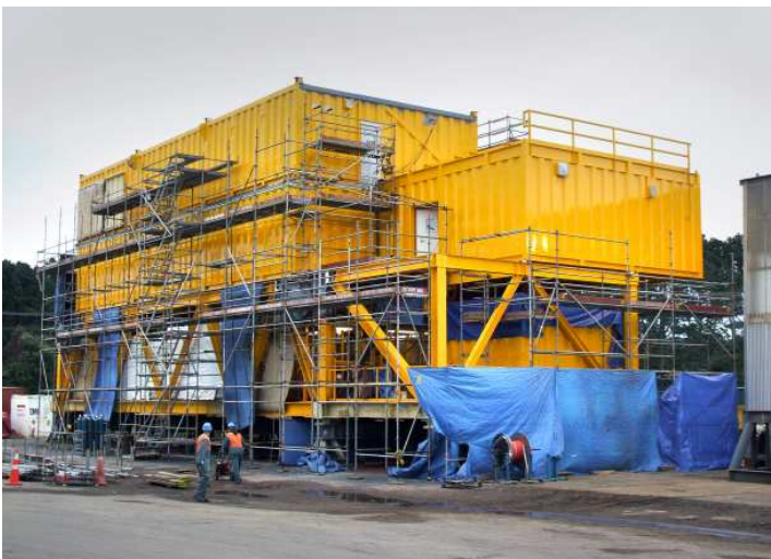
In 2009, Fitzroy won an over $30 million EPC project associated with a mid-life enhancement (MLE) programme for the offshore Yolla gas field platform in Bass Strait, Australia and crucial to this development is enabling the Yolla platform to accommodate project personnel. Fitzroy Engineering's contract is to manage, engineer, fabricate and deliver the new accommodation and utilities "megamodule" to the project. To be shipped in October 2011, this megamodule will be made up of nine units of various sizes and total transport weight will be approximately 630 tonnes. The entire unit will be transported from Fitzroy Engineering's New Plymouth fabrication yards to Port Taranaki and loaded on board a specialist transport vessel to the Bass Strait for installation.
