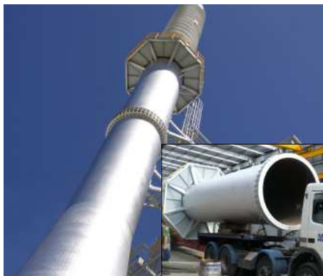
Flare Stack designed and built by HERA member Vortex Engineering for OI Glass expansion project in Penrose, Auckland. HERA member Grayson Engineering, fabricated the stack as part of a $1.2m contract involving approx 250 tonnes of support steel for the waste gas cleaning plant upgrade with the fitting of an Electrostatic Precipitator.
