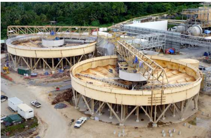
Two 48m grind thickeners and reagent infrastructure built by HERA member Tenix New Zealand for client Newcrest at their Lihir gold mine in Papua New Guinea. In addition, Newcrest also awarded packages to install 190 tonnes of pipe racks and also to install 9km of small bore piping and mechanical plant to the NCA tanks Tenix supplied the previous year.
