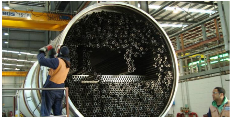
GEA Evap/Dryer NZ's $150 m work will include the world's largest yielding stainless steel dairy spray dryer. The second dairy spray dryer at the Darfield site will be capable of producing 30 tonnes per hour of milk powder from 4.4 Million Litres per day of milk. To keep the plant full will require milk from 260,000 cows."
