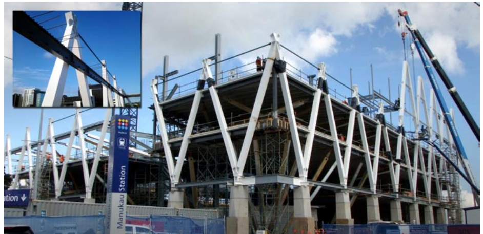
The MIT Campus and Transport Interchange building was a great example of pre-fabrication and collaboration. This amazing building over a live train station would have been near impossible without pre-fabrication. HERA members Holmes Consulting, MJH Engineering and Mainzeal are involved in the project.
