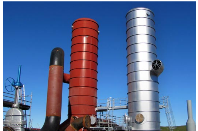
HERA member Tenix New Zealand fabricated these separators for client Contact Energy's Te Mihi power station
