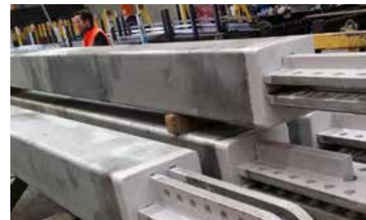
| Top | Alan McClintock working on 'k-area project' - welded hot rolled sections | Bottom | Research done at SFC certified fabricator D&H to identify key impact factors affecting quality welds
