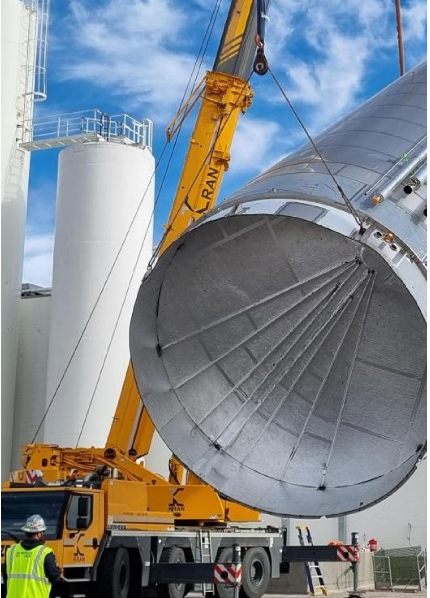
Milk silo install in the USA. Fabricated on site by Tira spiral welding technology
